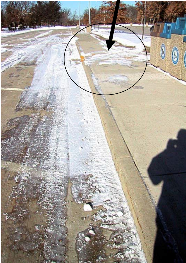
Does Not Meet Standards
